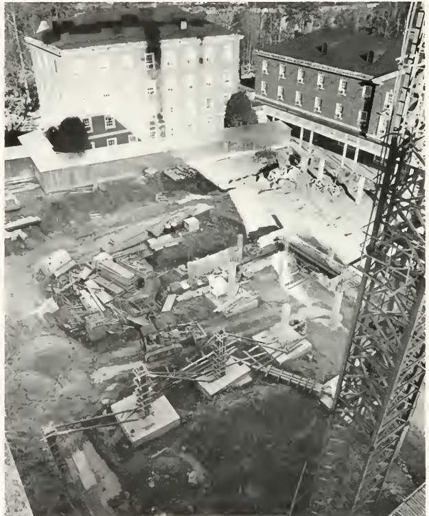
Progress on the patient support facility pictured here that will house the Burn Center is expected to be completed in about two years.
